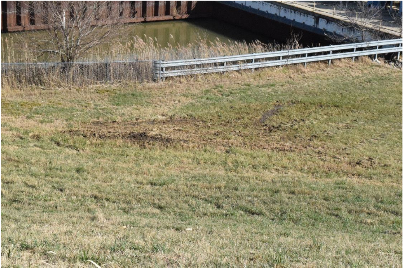
East side seepage at toe – observe this area
